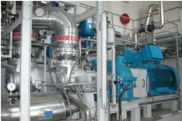
Screw-type steam engine (730 kWel) in the Hartberg biomass CHP plant; Cooperation project with the University of Dortmund (Germany)
