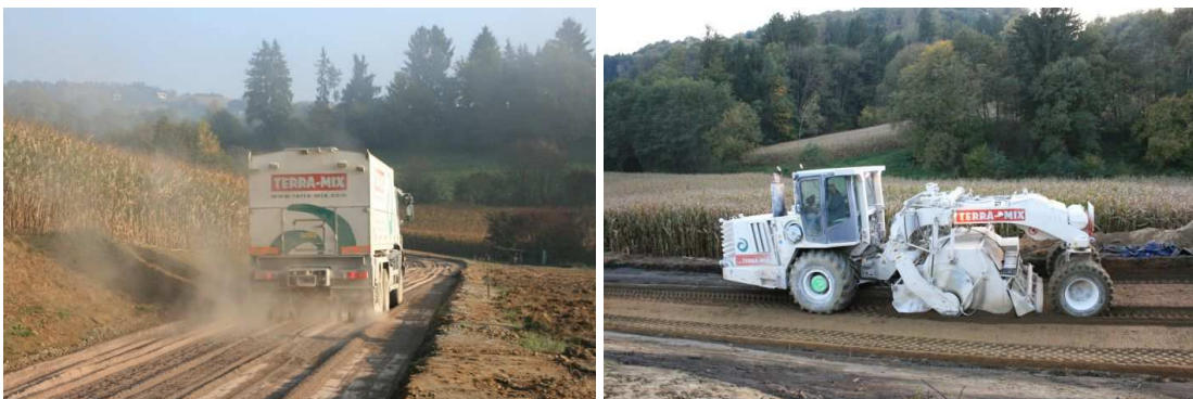
Construction of a new road section with wood ash as stabilising material in Styria
