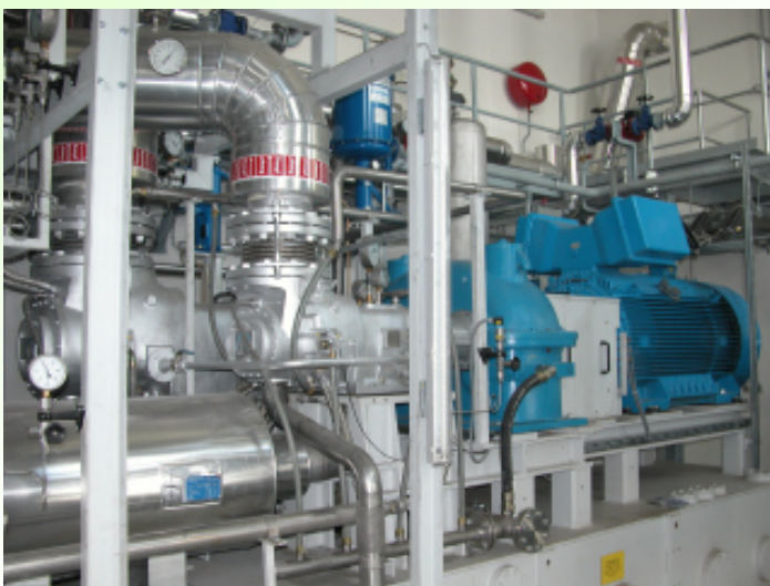
Screw-type steam engine (730 kW el ) at the biomass CHP plant Hartberg (A)
